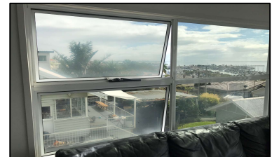
Figure 3: Interior window film applied to casement windows, that turned milky/cloudy over time from being exposed to outside elements.
