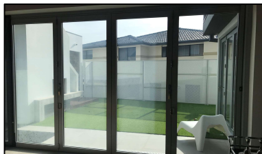
Figure 1: Hardcoat breakdown of an interior window film that was applied to bifold doors.
