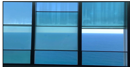
Figure 2: Vertical sliding windows right off the water that exposed an interior window film to significant moisture/condensation, causing the hardcoat to break down.
